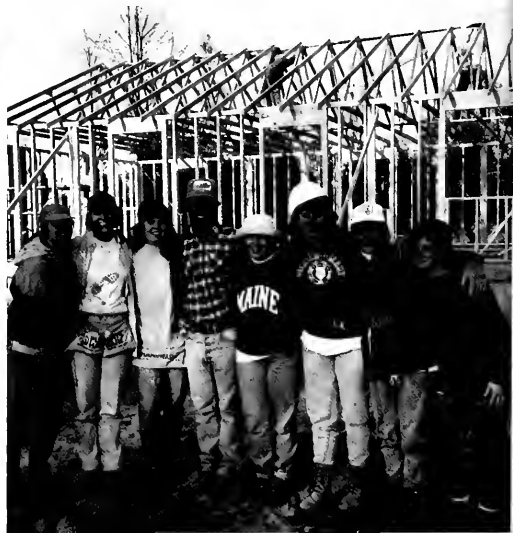
Great build! Berna, Caroline, Terri, Jon, Amelia, Lori, Sarah, and Tracy pose in front of the house they're building for Habitat for Humanity.
